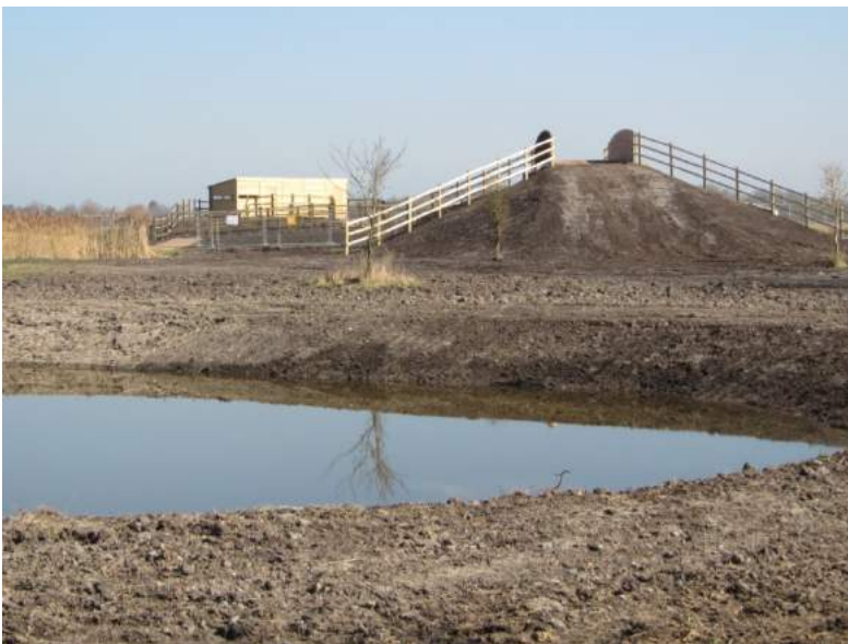
The finished Harrison's Drove bridge and the new hide seen from the south (Harrison's) side. The hide overlooks Baker's Fen and one of the larger pools. New ponds have been created where soil was excavated to build the ramps.
