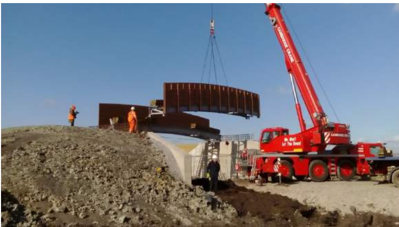
The huge crane manoeuvres the Harrison's Drove bridge side sections into place, in February 2016.
